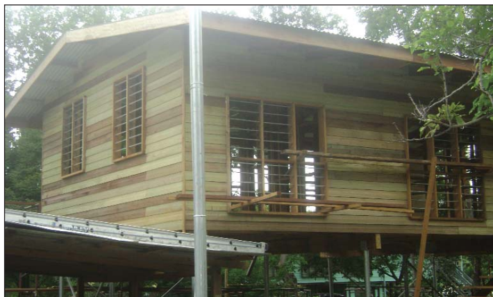
• This is one of the three bed room houses under construction at Kanudi estate in Port Moresby. (Picture by Steven Poning)
